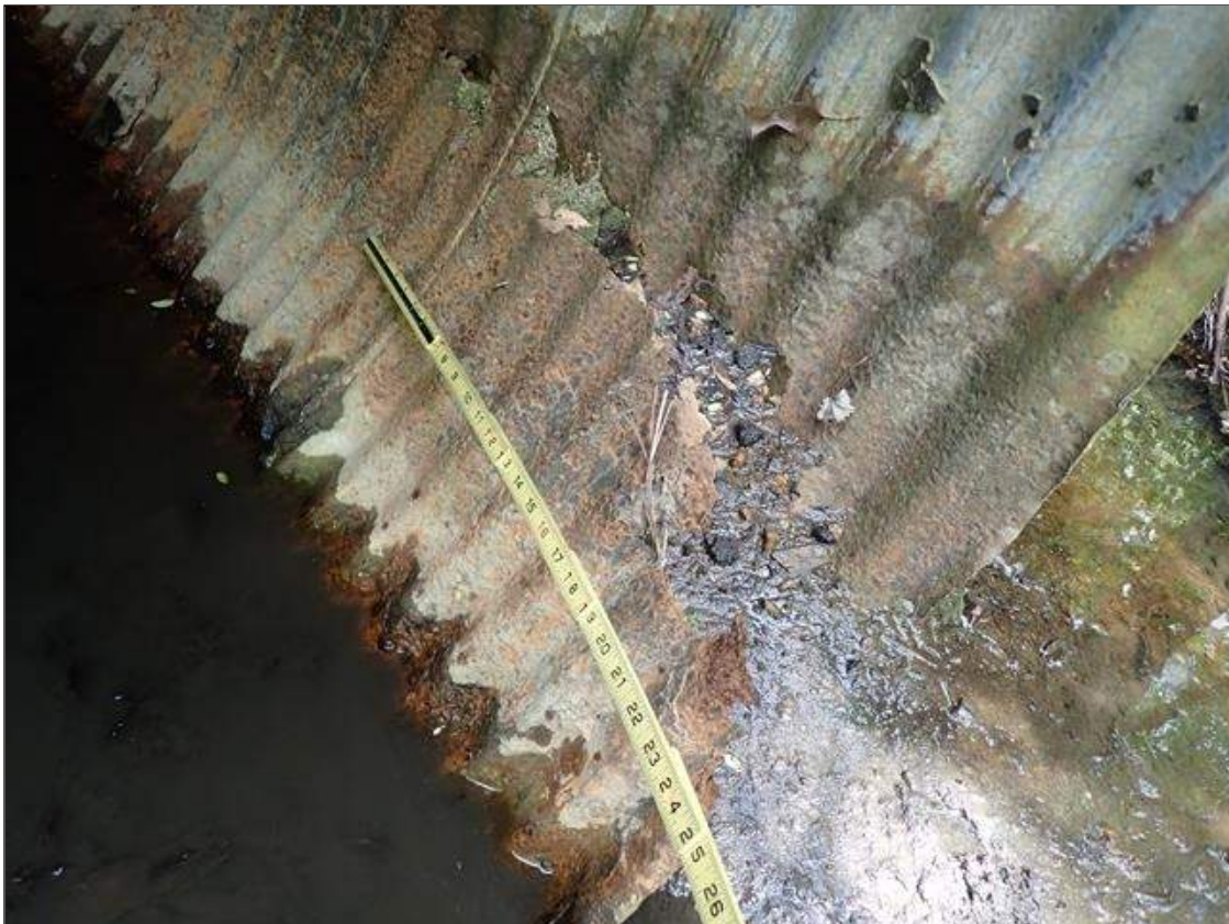
Span 2 Section 3: (PAR Municipal) at downstream end of pipe extending past headwall, on east side, corrosion with 100 percent section loss (24 inches x 8 inches) with rust scale surrounding
