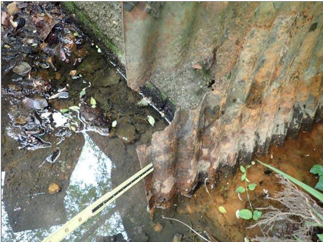
Span 3 Section 3: (PAR Municipal) at downstream end of pipe extending past headwall, on east and west sides, corrosion with 100 percent section loss (up to 27 inches x 7 inches) with rust scale surrounding
