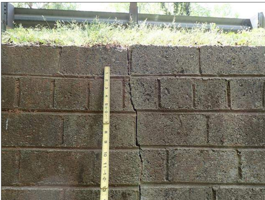
north headwall above barrel 3, vertical crack (full height x 1/8 inch wide)
