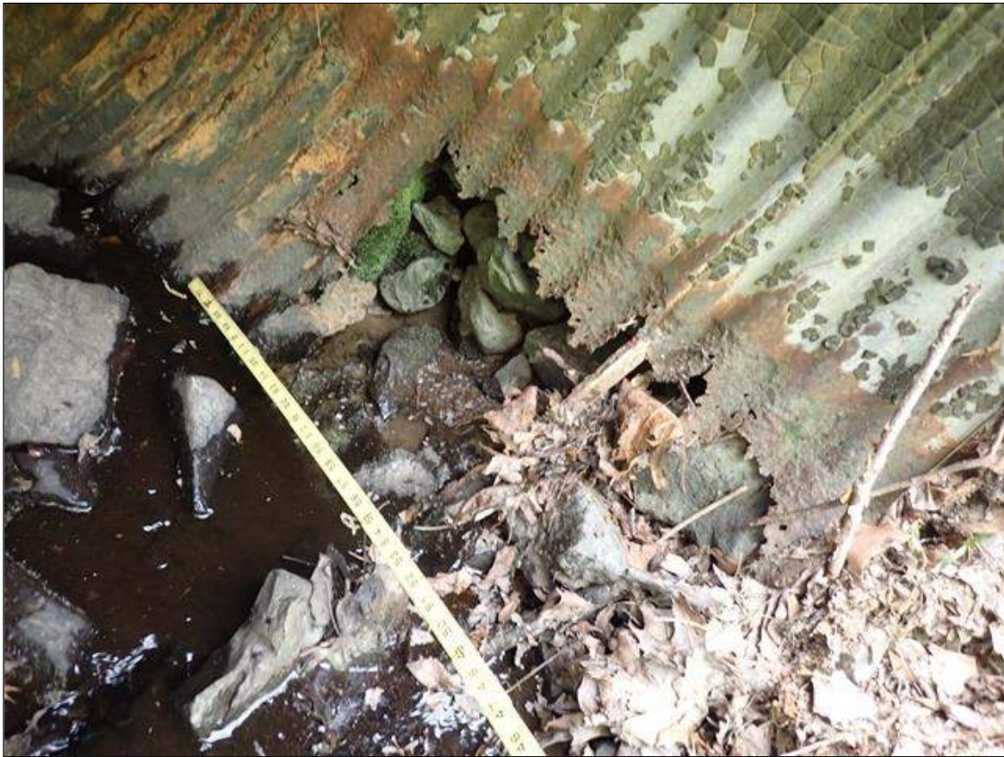
Span 1 Section 1: (PAR Municipal) upstream end of pipe, outside headwall on east and west ends, corrosion with 100 percent section loss (up to 31 inches long x 12 inches high) with rust scale on adjacent steel
