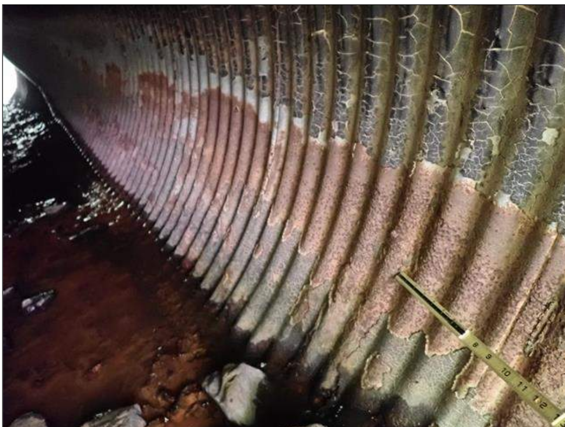
Span 2 Section 1: bottom third of barrel throughout segment, rust scale and loss of tar coating
