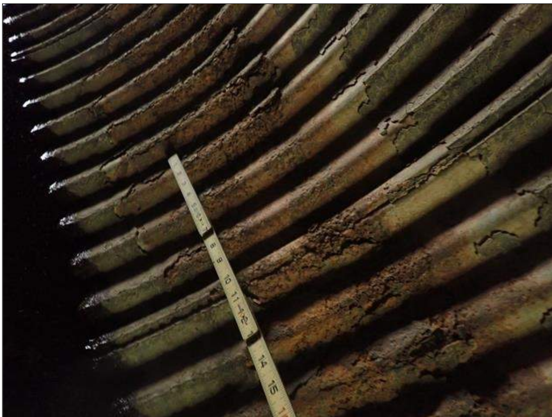
Span 1 Section 2: bottom third of barrel throughout segment, rust scale and loss of tar coating
