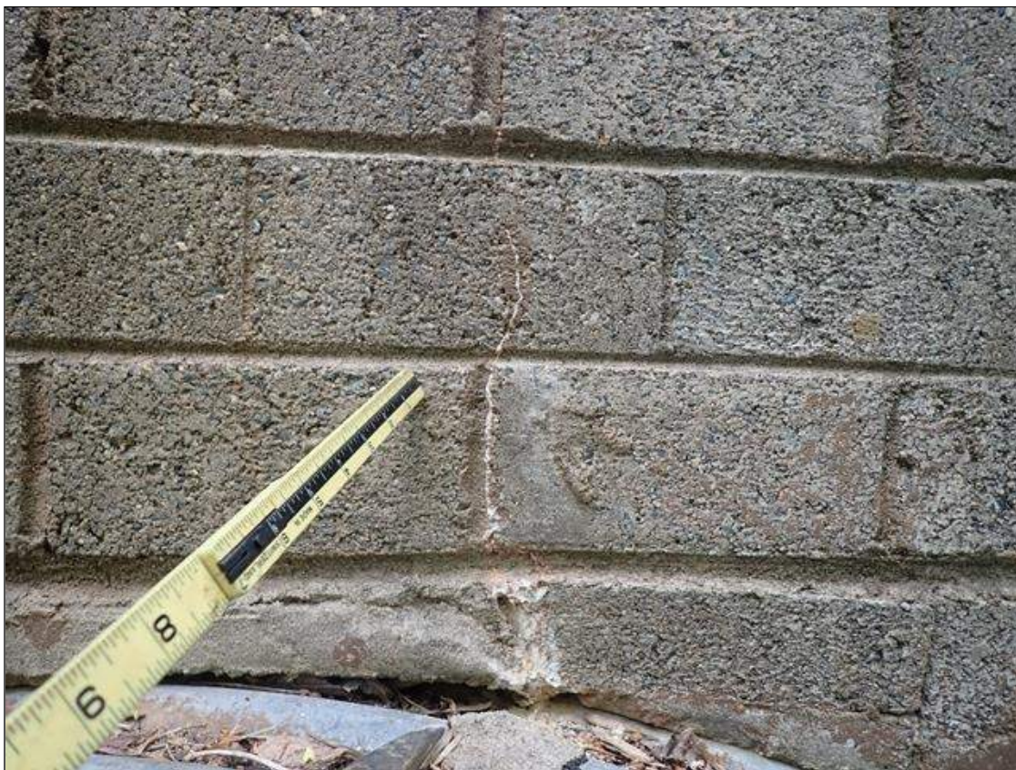
south headwall above barrel 2, (2) vertical cracks (full height x up to 1/32 inch wide) with efflorescence
