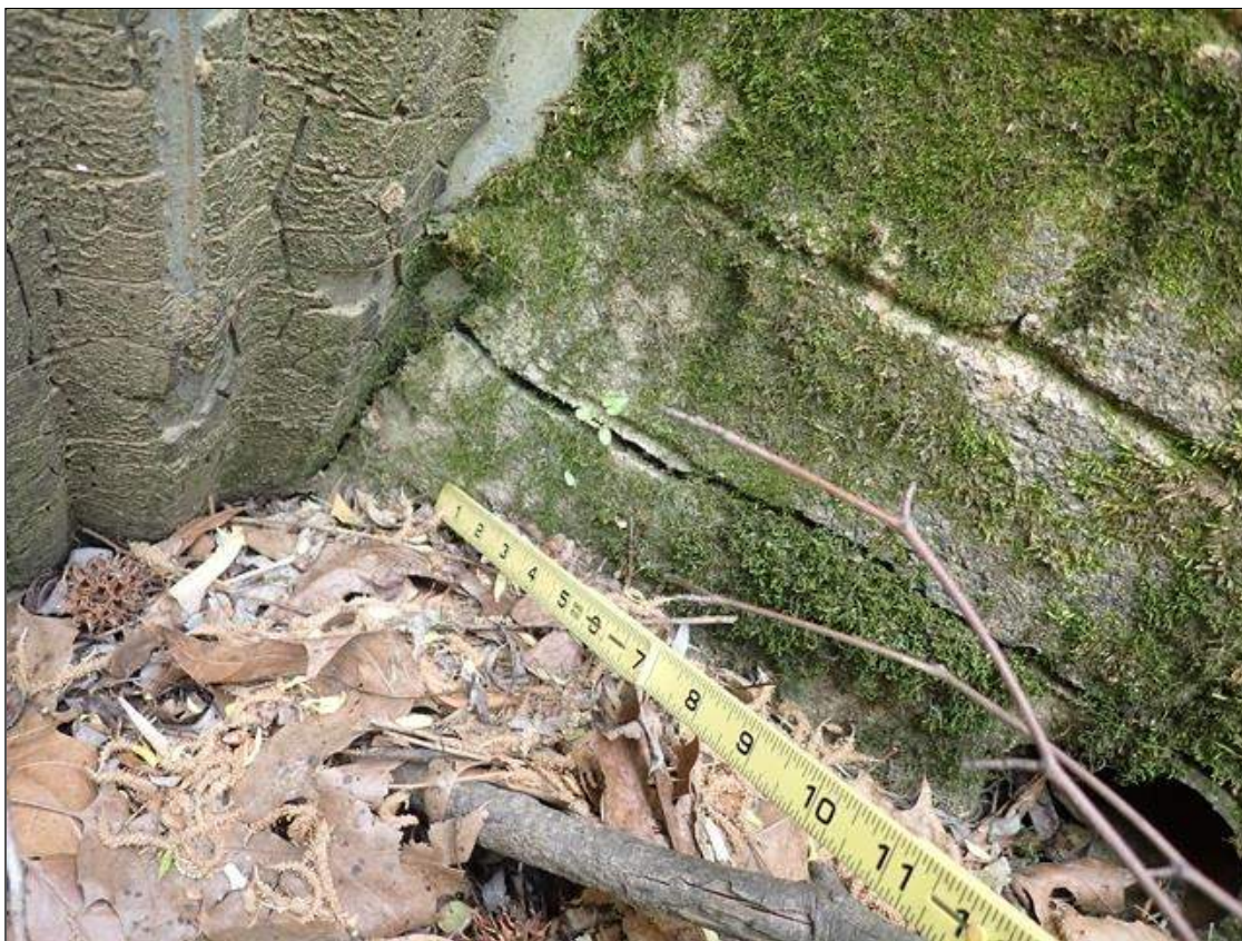
north headwall between barrels 2 and 3, horizontal crack (1/16 inch wide)
