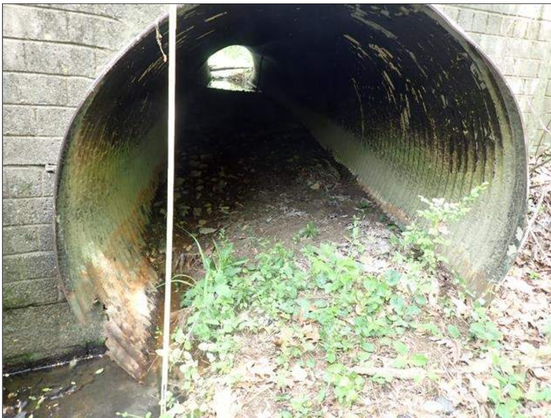
in barrel 3, sediment buildup (up to full length x 5 feet x 1 foot)
