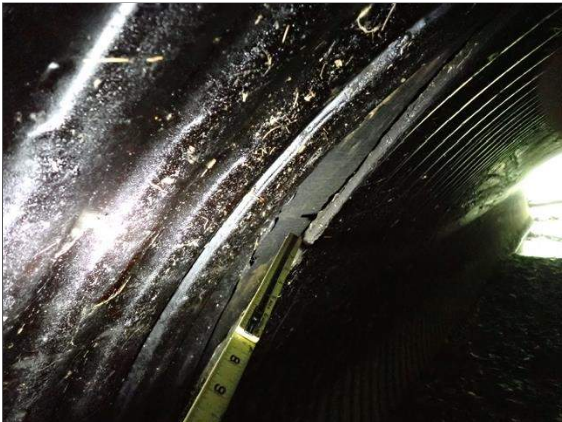
Span 3 Section 2: (PAR Municipal) joint of sections 2 and 3, offset (up to 2 inch) with connection band visible and fill visible at end of band
