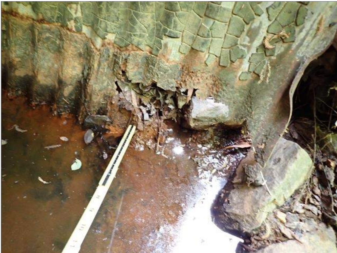
Span 3 Section 1: (PAR Municipal) at upstream end of pipe extending past headwall, on west side, corrosion with 100 percent section loss (17 inches x 10 inches high) with rust scale surrounding
