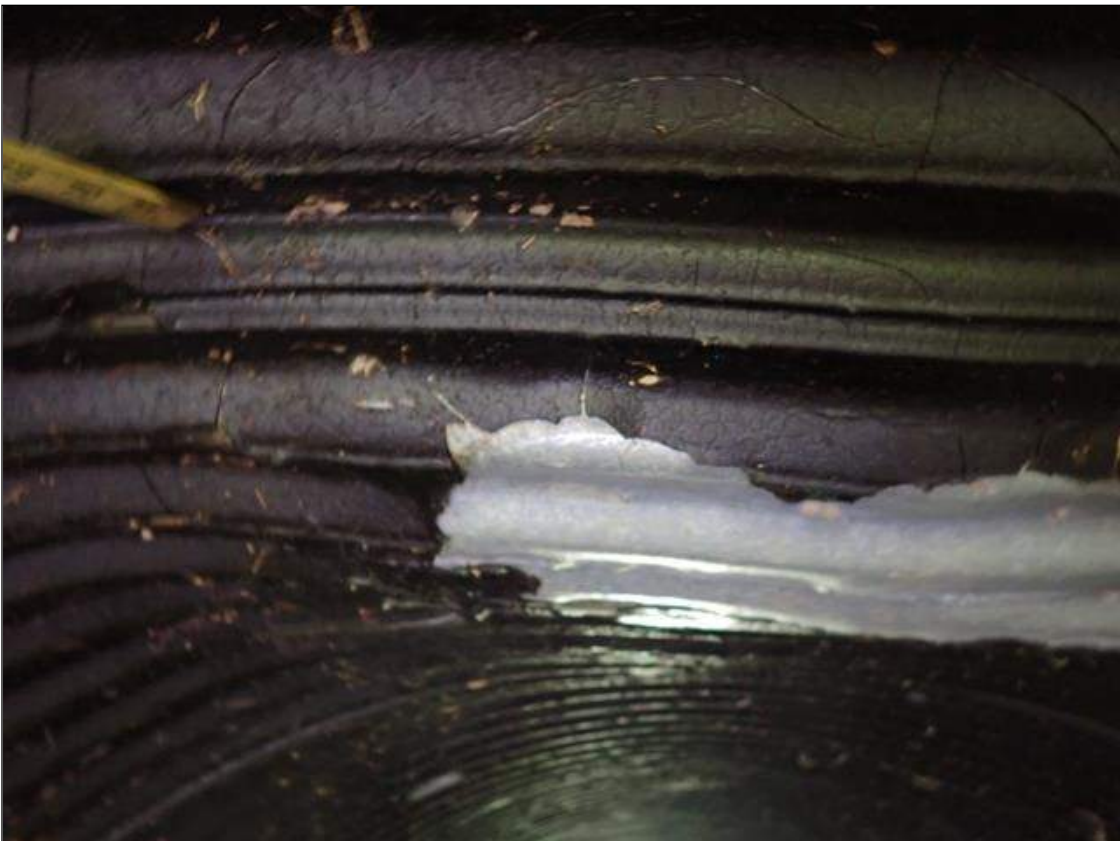
Span 1 Section 3: in top of barrel 7 feet from downstream end, bulge (36 inches x 18 inches x 3 inches deep) at 11 o'clock position with missing tar coating
