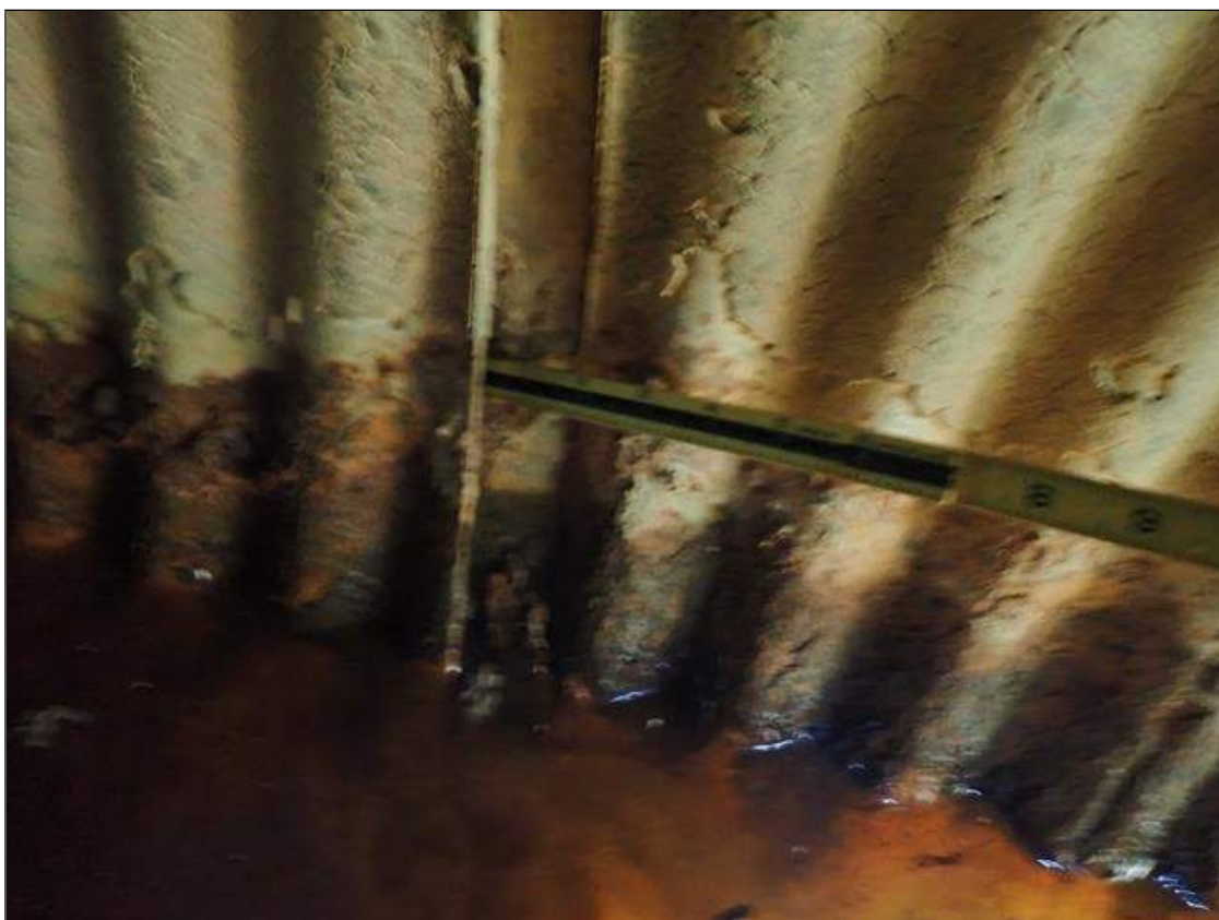
Span 3 Section 1: in joint of segments 1 and 2, distortion (up to to 1.5 inch)
