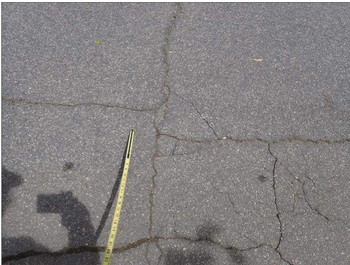
asphalt over barrels, scattered map cracks (up to 1/16 inch wide)
