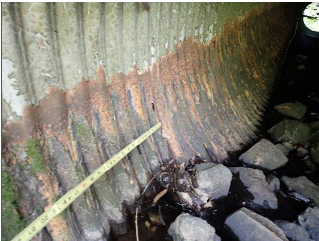
Span 1 Section 1: bottom third of barrel throughout segment, surface rust and loss of tar coating
