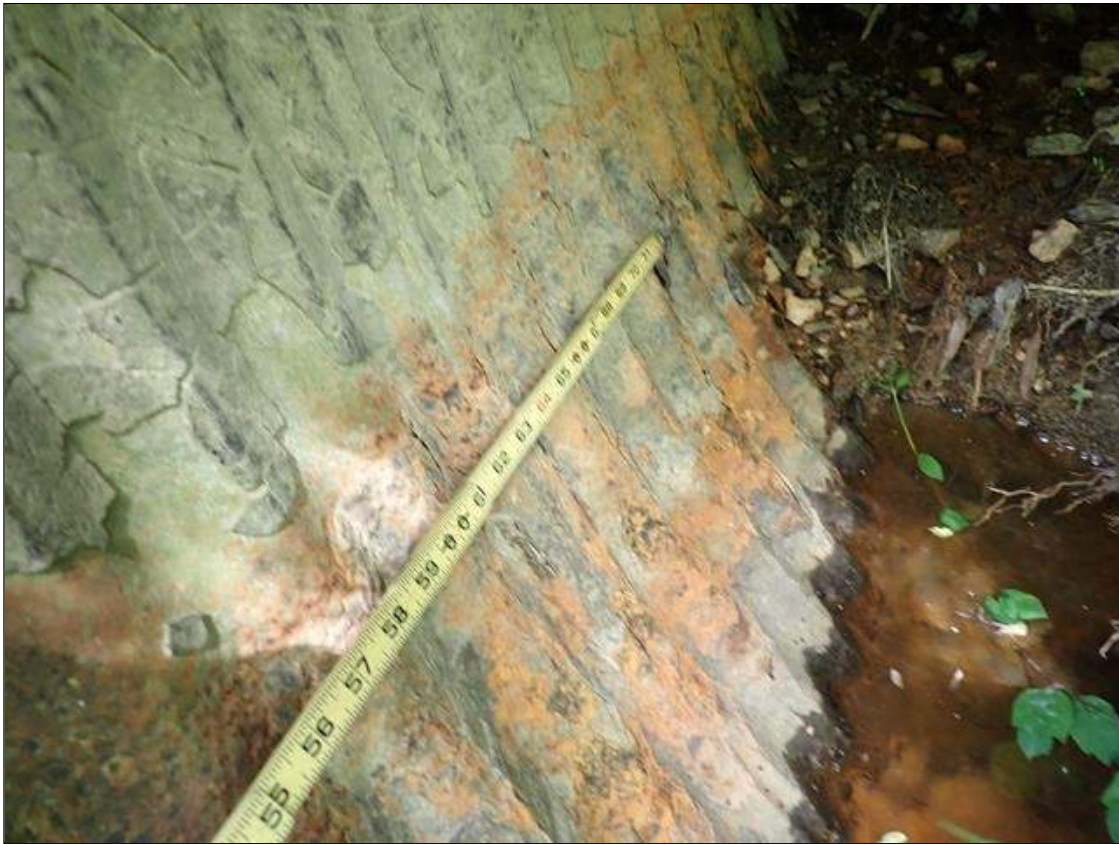
Span 3 Section 3: bottom third of barrel throughout segment, rust scale and loss of tar coating
