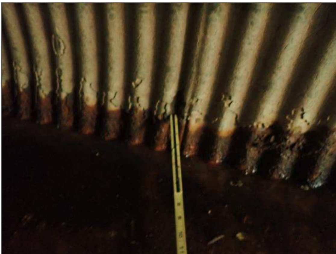
Span 3 Section 2: bottom third of barrel throughout segment, rust scale and loss of tar coating
