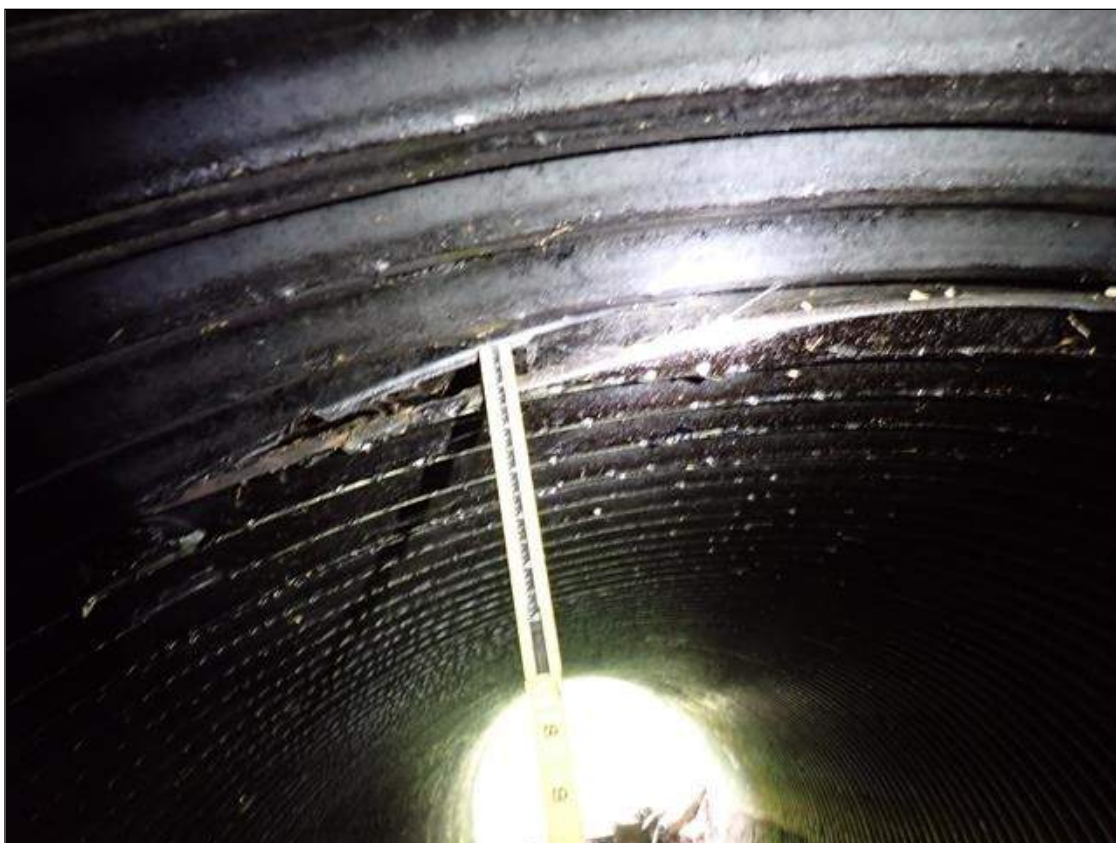
Span 2 Section 1: at 12 oclock position at end of segment, distortion (up to 4 inch)
