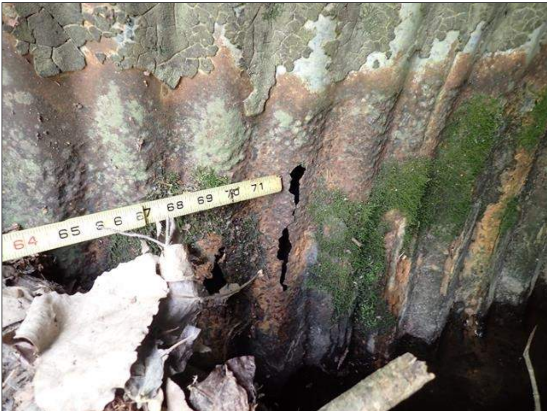
Span 1 Section 1: (PAR Municipal) upstream end of pipe, outside headwall on east and west ends, corrosion with 100 percent section loss (up to 31 inches long x 12 inches high) with surface rust on adjacent steel
