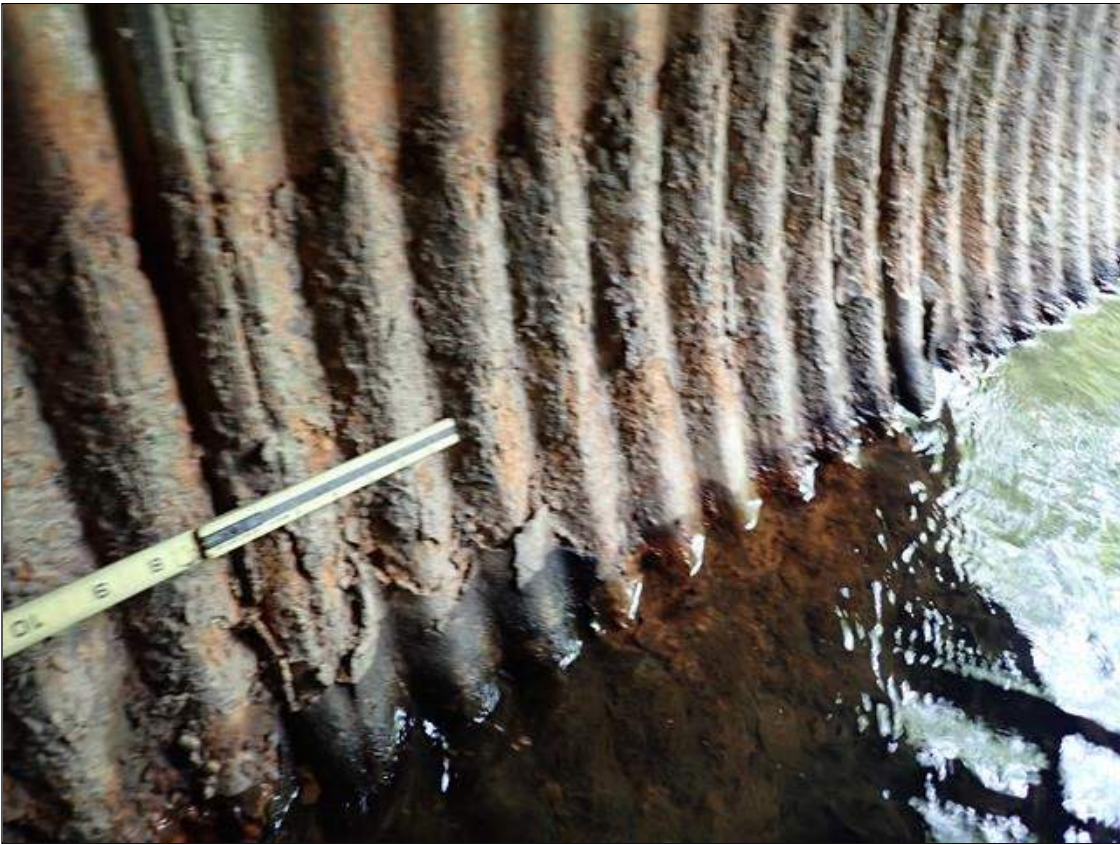
Span 2 Section 3: bottom third of barrel throughout segment, rust scale and loss of tar coating
