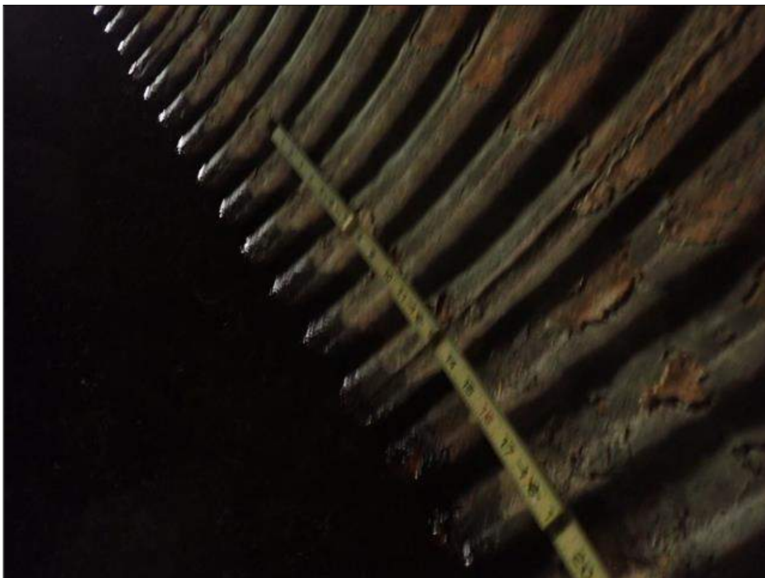
Span 2 Section 2: bottom third of barrel throughout segment, rust scale and loss of tar coating
