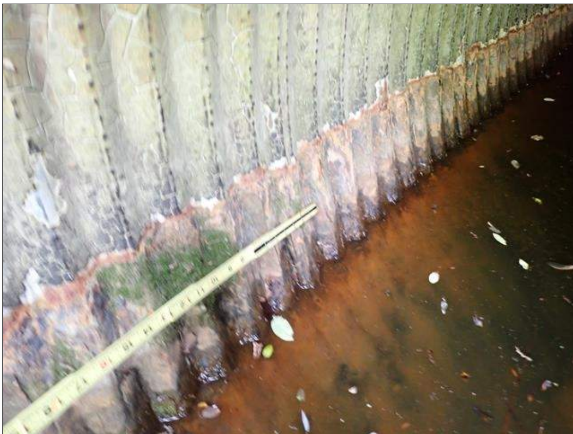
Span 3 Section 1: bottom third of barrel throughout segment, rust scale and loss of tar coating
