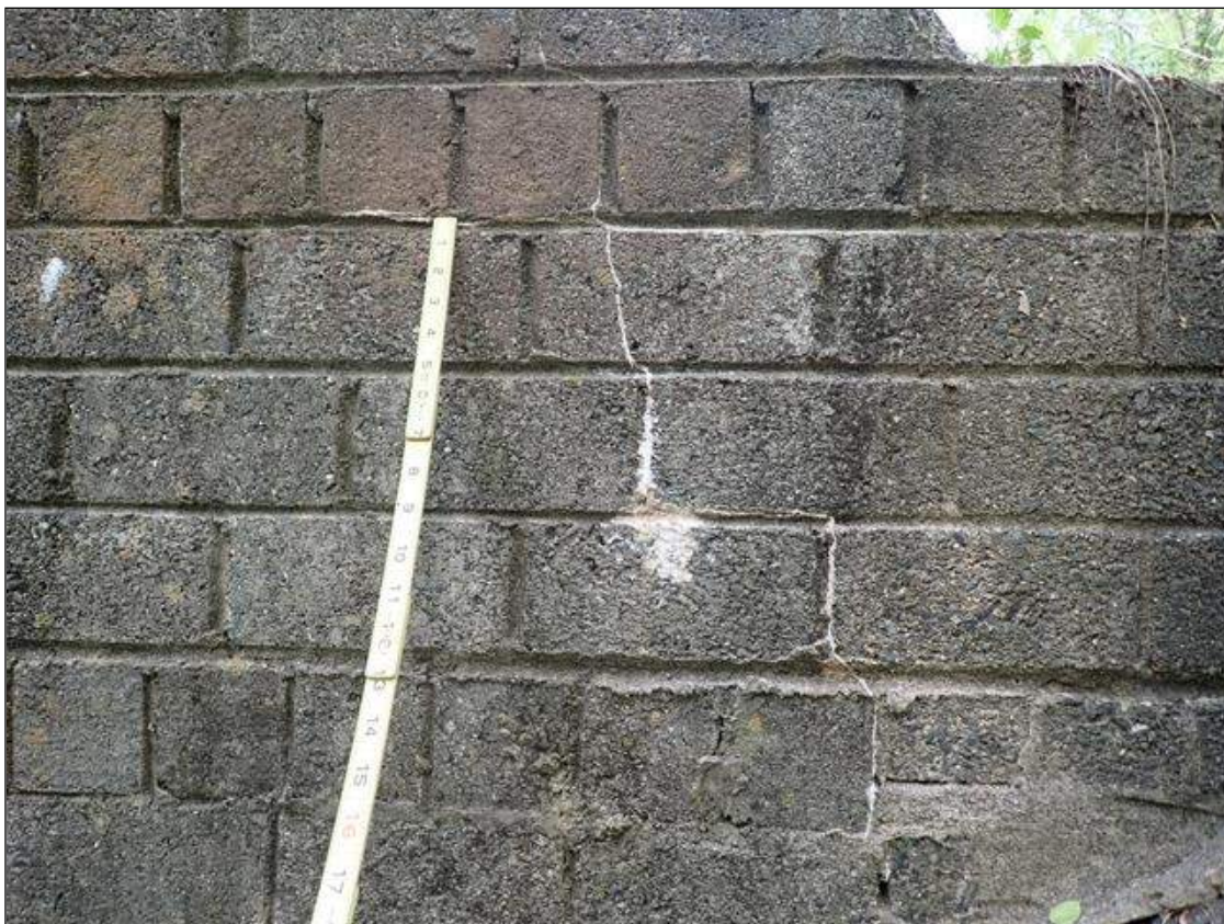
south headwall over barrel 3, scattered vertical cracks (1/32 inch wide) with efflorescence
