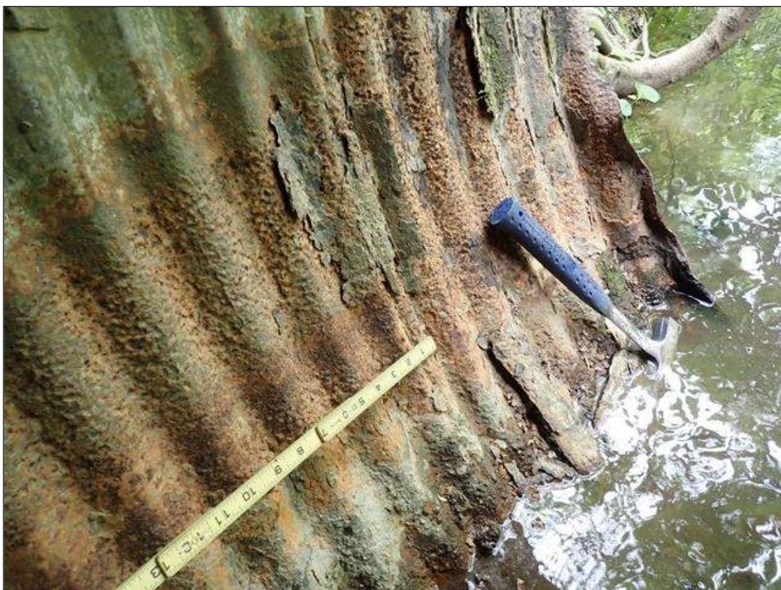
Span 1 Section 3: bottom third of barrel throughout segment, rust scale and loss of tar coating
