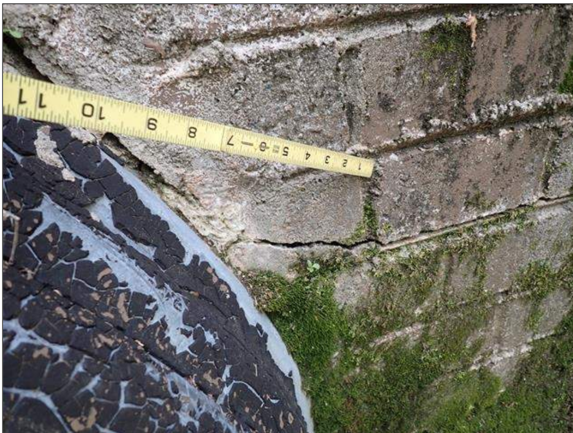
north headwall between barrels 1 and 2, horizontal crack (up to 1/16 inch wide)
