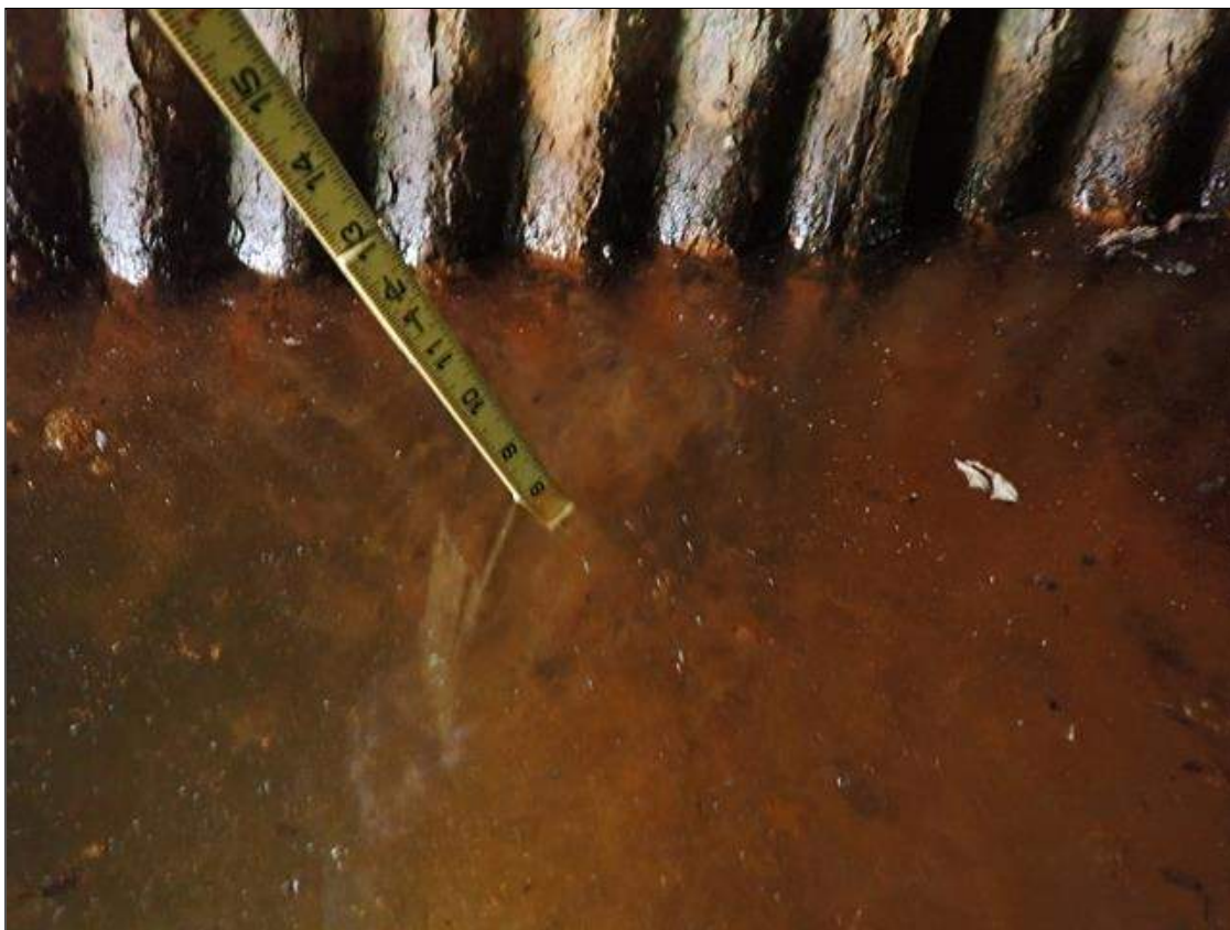
Span 3 Section 1: end 1 inch on east side at upstream end has 2 inch diameter hole (under water at time of inspection)/AREA OBSCURED BY WATER 4/6/22
