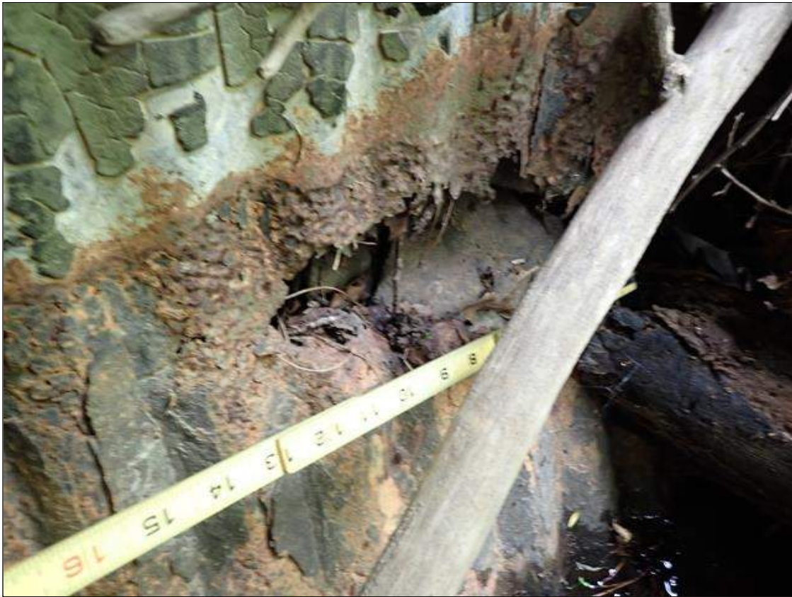
Span 2 Section 1: (PAR Municipal) upstream end of pipe, outside headwall on east and west ends, corrosion with 100 percent section loss (up to 15 inches long x 5 inches high) with rust scale on adjacent steel
