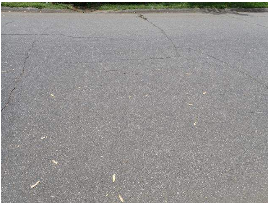
asphalt over culvert
